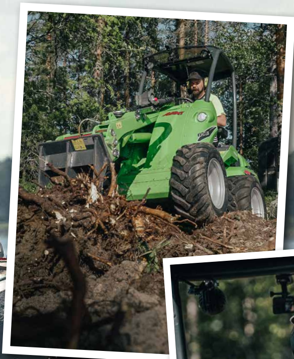
Stumps getting rough treatment from the Ripper and Janne Kaperi. Below, Kaitsu Rinkinen behind the wheel.
